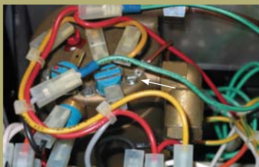
Fig. 1 Thermocouple washer installed under screw of steam thermostat.
