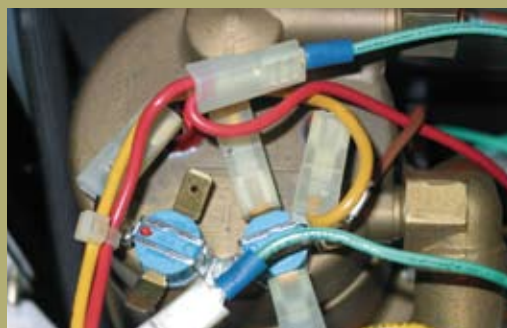
Fig. 3 Boiler detail with thermocouple and SSR wires installed.
